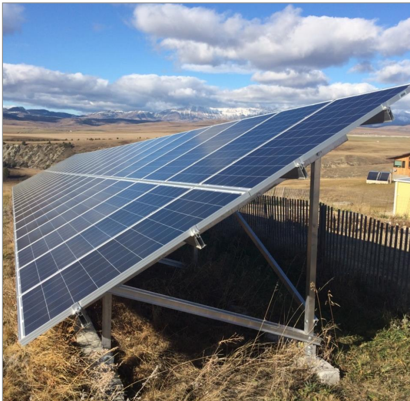
Rural Microgeneration Project Providing Surplus Energy into the Grid, Photo by M. Neville
